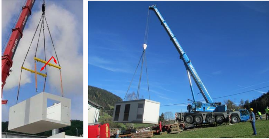
Fig. 19: Installation with and without a roof
