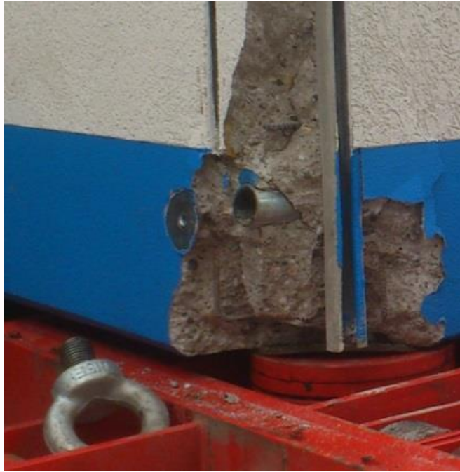
Fig. 8: Deformation caused by a prohibited lifting method
